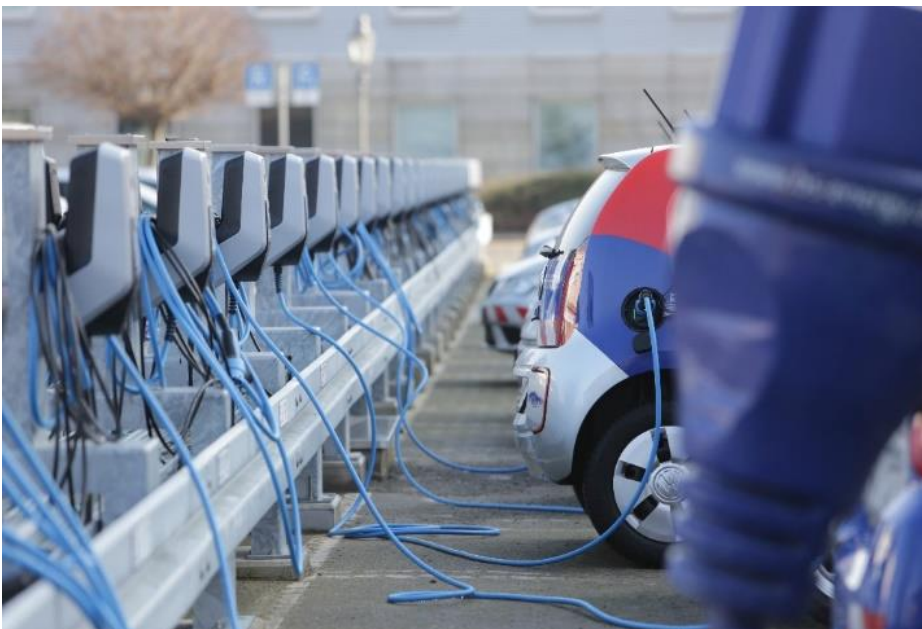
Fuhrpark BS Energy in Braunschweig
